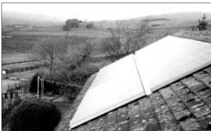
A solar PV system helps to reduce electricity bills at this youth hostel during its busiest period, between March and October. Photo courtesy of Windsund International.
